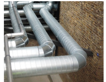
Ductwork, Ventilation and Heat Recovery
